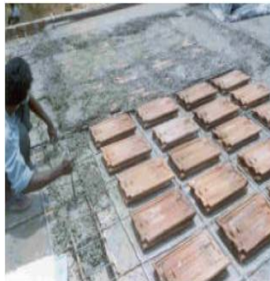
Fig: 13. Photograph shows the arrangement of Mangalore tiles.
