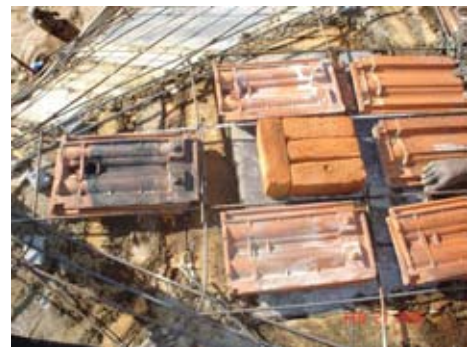
Fig: 14. Photograph shows the arrangement of Mangalore tiles.
